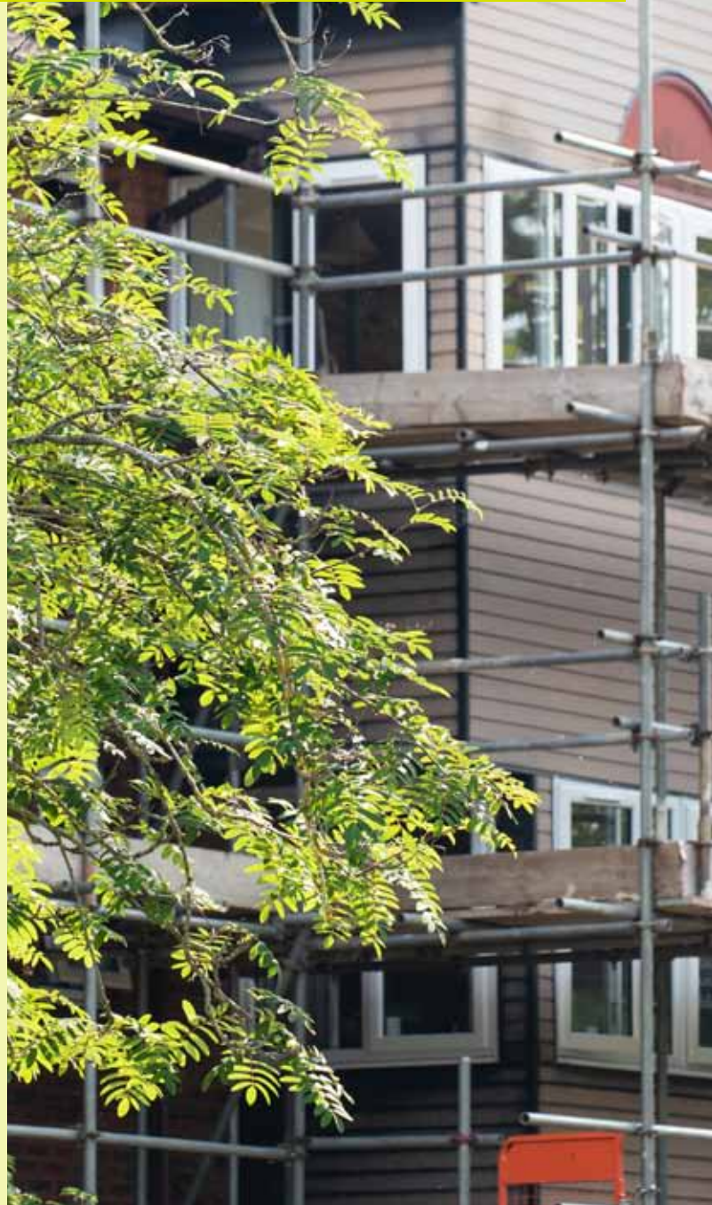
Improvement work is underway at Flowerpot Lane with windows and fascias being renewed
