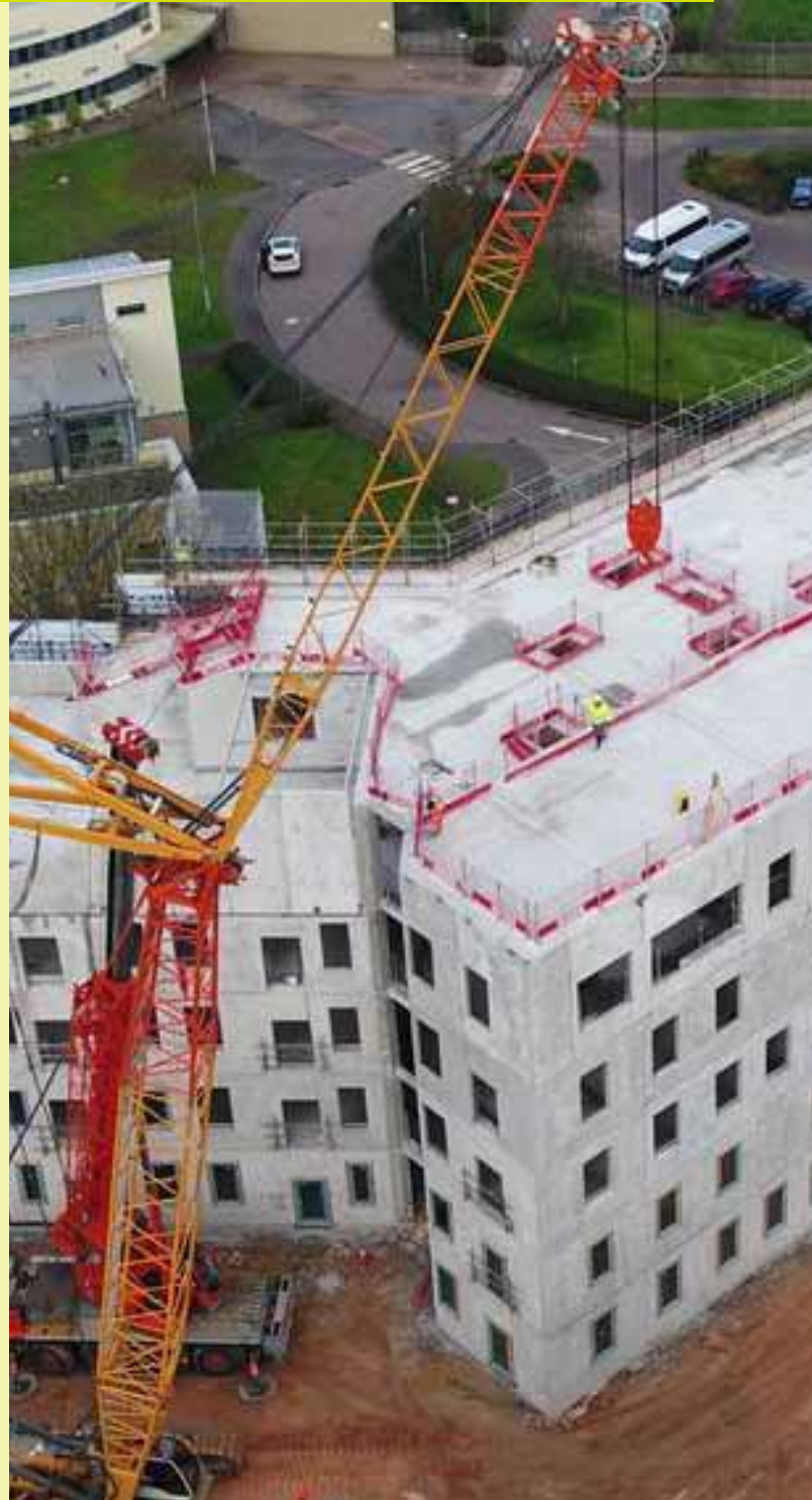
Construction is well underway at the Edwards Court Extra Care Scheme on Topsham Road.
